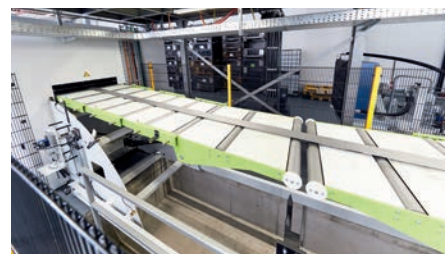
The strip is transferred to the downstream press or punching machine via a loop pit with a radius of 2,000 mm. If required, the strip can be transferred horizontally via a strip transfer table.
